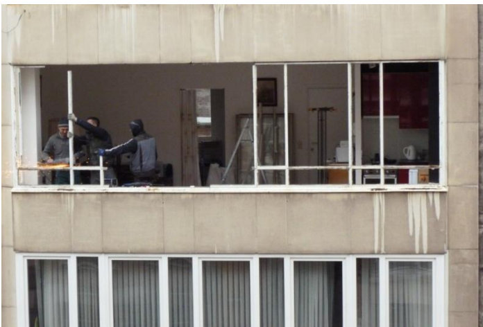
Figure 3: Destruction of original windows by cutting.
