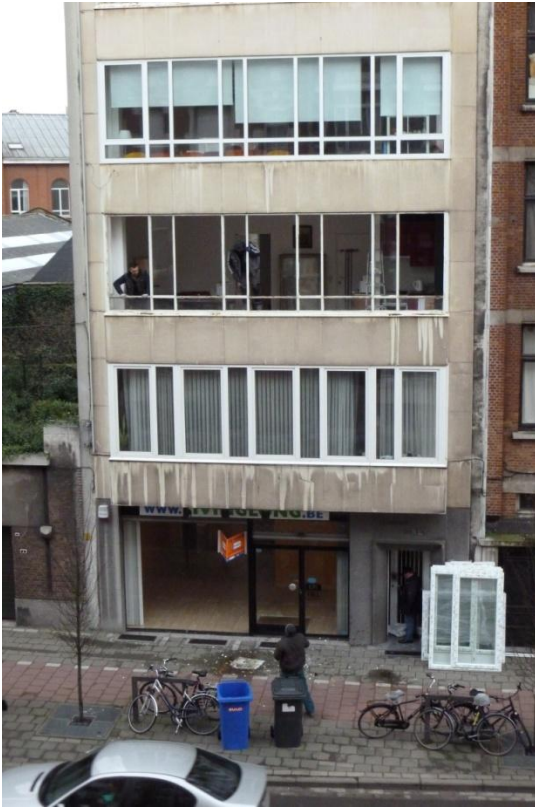
Figure 2: Destruction of original windows by hammering.
