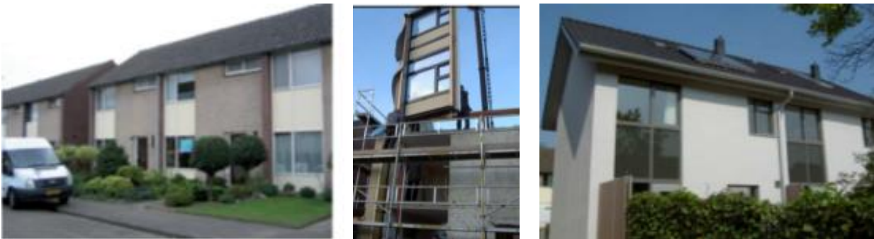
Figure 8: Prefab renovation of a housing estate in Roosendaal, the Netherlands (visited with Flemish One Stop Shop user group 08-09-2011). Left: houses before renovation; mid: prefab façade system used during renovation; right: after renovation. Source: IEA SHC Task 37.
