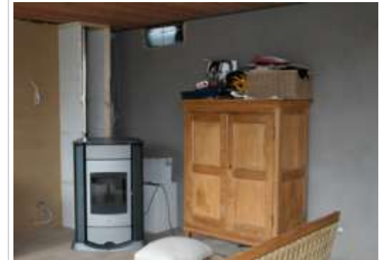
Pellet stove in the living room
