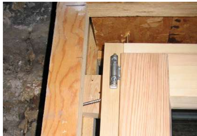
New passive window installed in the surface of the new timber construction
